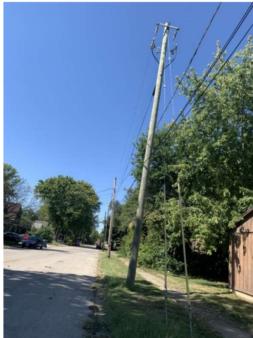
Project Transmission Line, Looking West on West River Street Near South 3 rd Avenue
