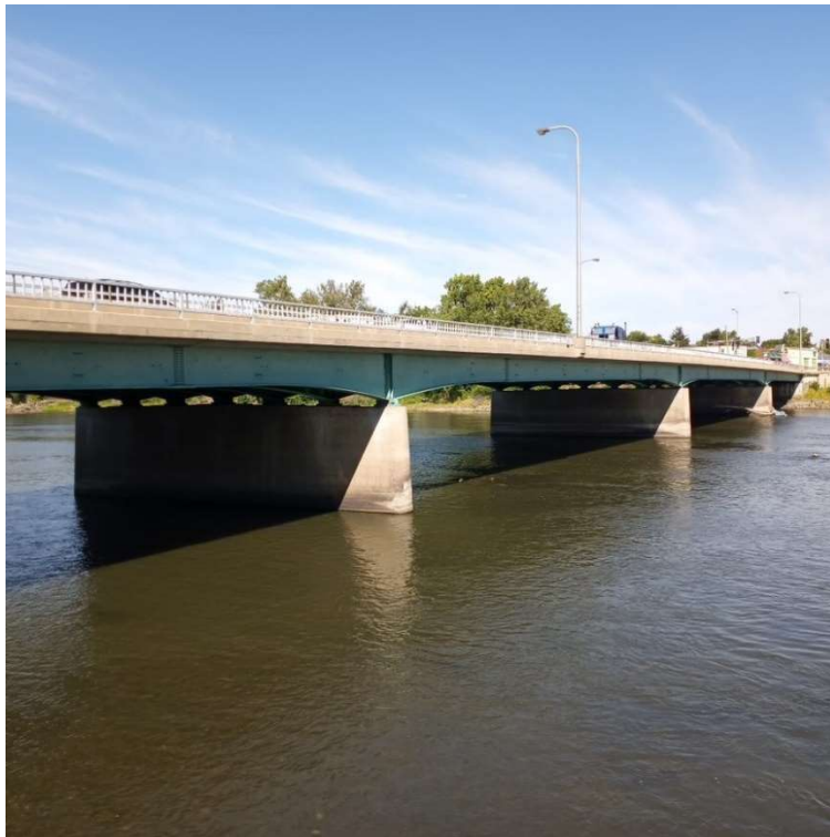
South McMullen Drive Bridge (Includes Project Transmission Line Crossing of River in Conduit), Looking Northwest from Tailrace Fishing and Viewing Area
